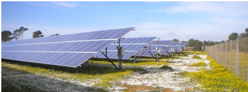
Anlage Lluçmajor, Mallorca, 1.775 MW
